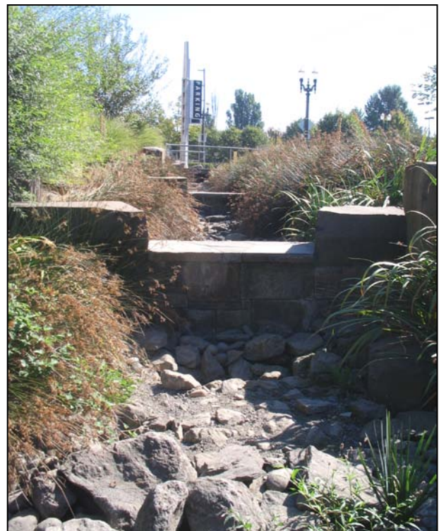
Check dams in this swale slow erosive flows
