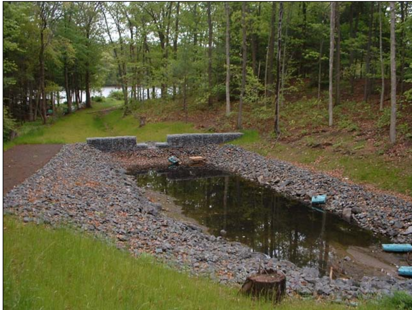
Eroded stormwater outfall on lake replaced with infiltration basin and vegetated swale.
